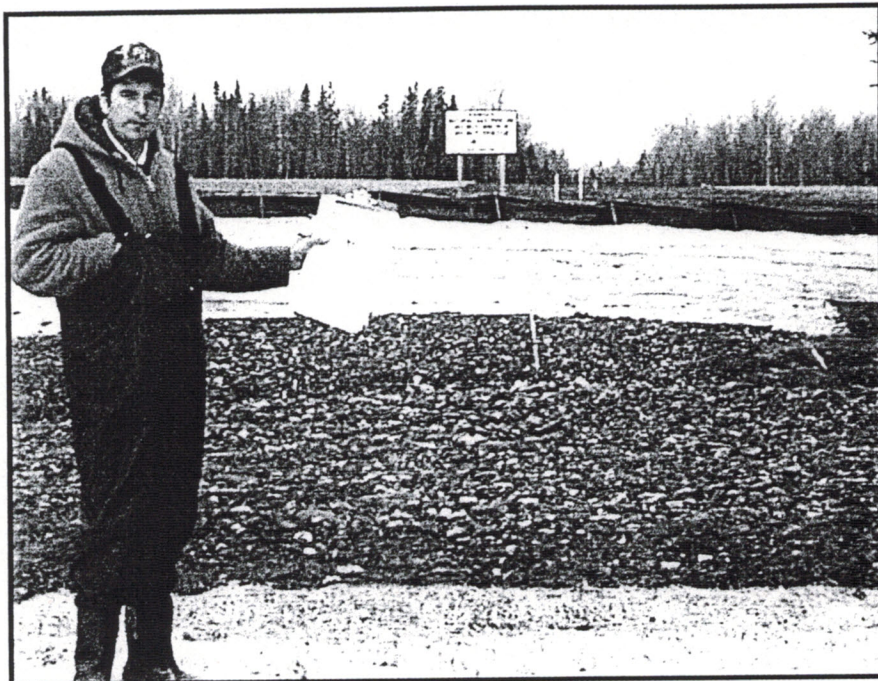
Figure 15. Pipeline construction at site 17.1 is leaving portion of land with no vegetation.
