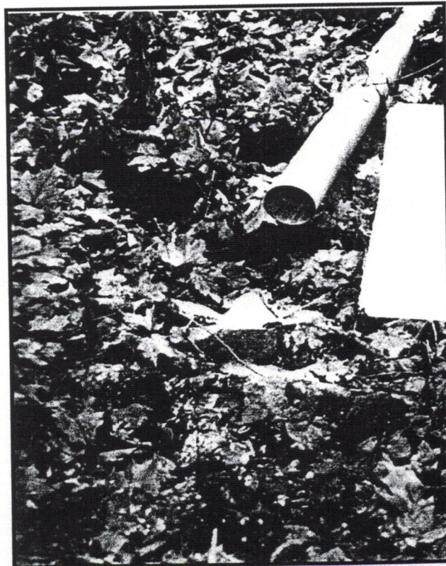
Figure 6. Plastic drainage pipe originating from a house at site 9.
