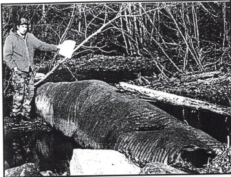
Figure 23. Rusting culvert pipe (abandoned) lying across a portion of the river at site 28.
