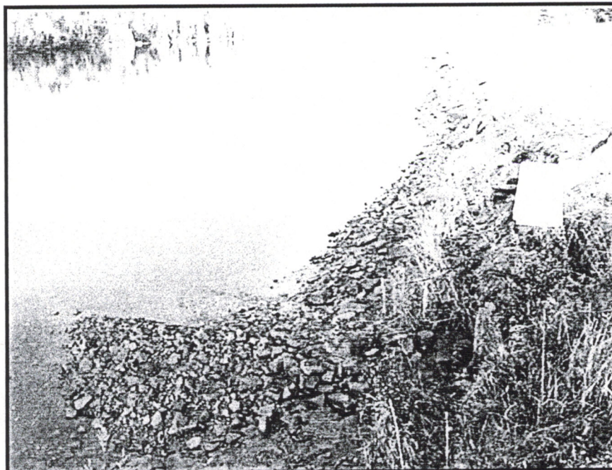
Figure 2. Serious erosion problems near culvert crossing dirt road at site 5.
